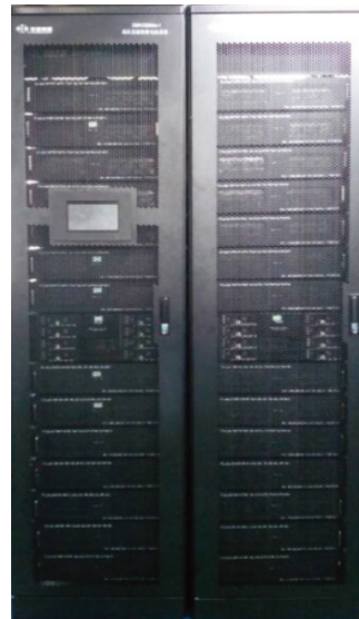
Fig. 1 336V/200Ah high voltage DC lithium-ion battery system for telecommunication
