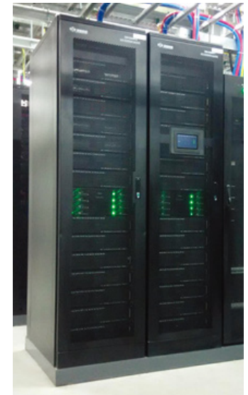
Fig. 2 high voltage DC lithium-ion battery system for telecommunication in China Harbin Mobile IDC application scenarios
